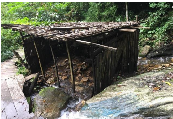
Figure 15: Plates 15 - Dilapidated shed for relaxation
